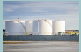
Tank to Tank
