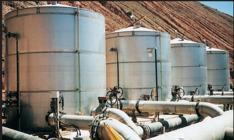
Four of sixteen 12,000 gallon T-316L stainless steel tanks for acidic leach solution in mining operations for Bechtel Corp.
